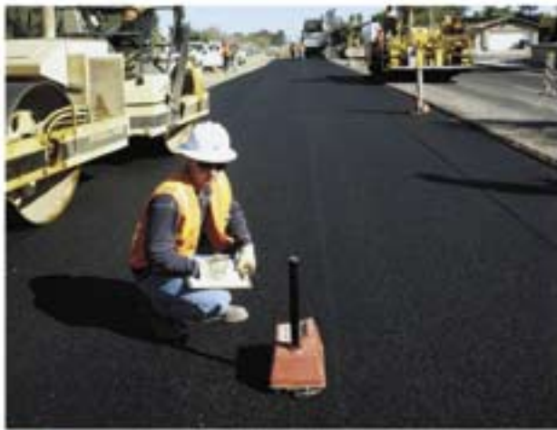
Asphalt testing at a City of Phoenix roadway construction project. HA assists the Contractor to develop their rolling pattern then provides the owner with QA testing to verify and document that the end product meets project specifications.
