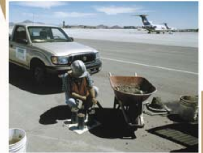
HA has performed QA and QC testing on numerous projects at Sky Harbor International Airport. Here HA collects concrete cylinders to verify compressive strength of concrete used to construct a new blast wall following relocation of the Air National Guard.
